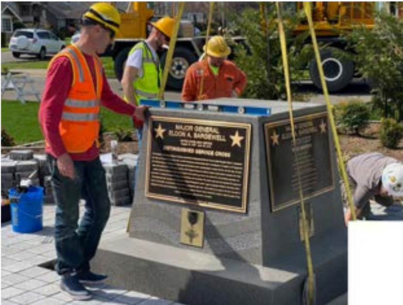
Workers install the base for the bronze sculpture of Major General Eldon Bargewell in Hoquiam
